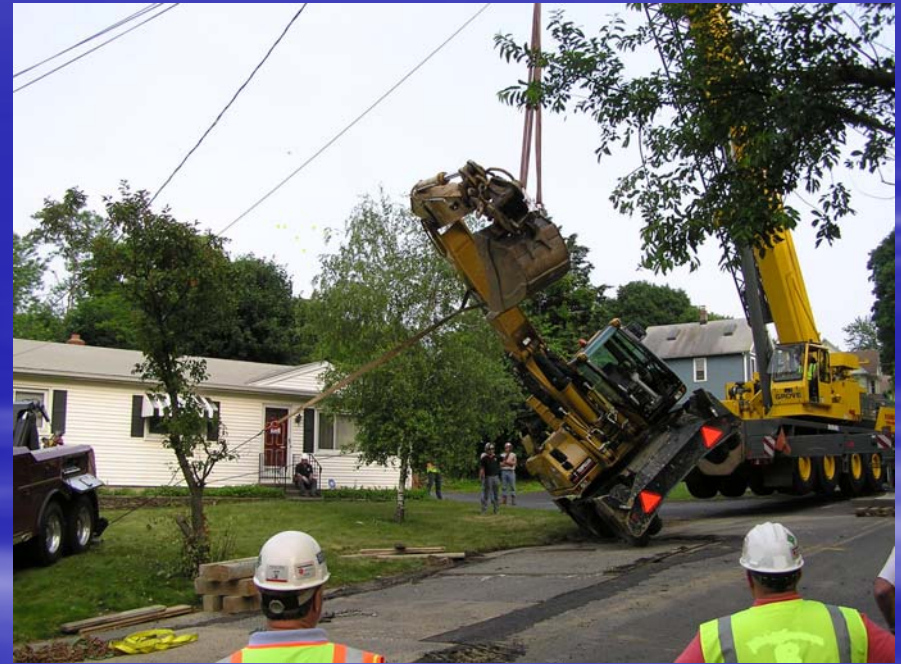
Rubber tire excavator flip over
