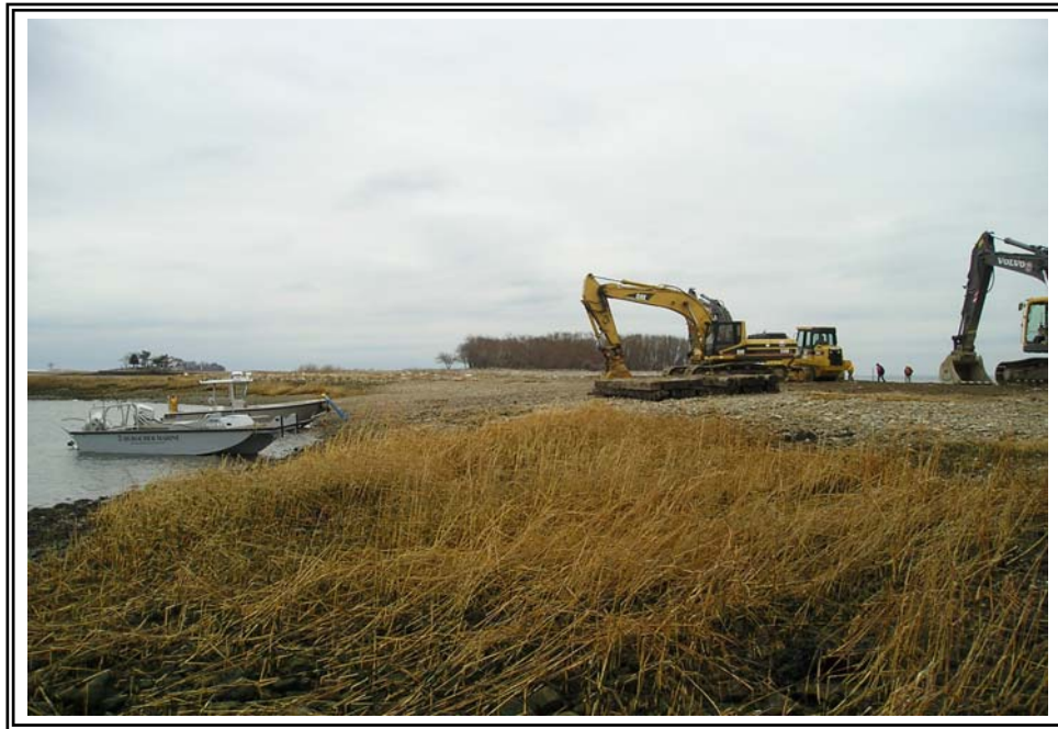
Photo 4: Photograph showing cable corridor immediately after cable burial. Extensive Spartina beds present east and west of cable corridor are clearly visible.
